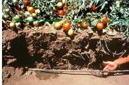
Installation of SDI system for tomatoes
